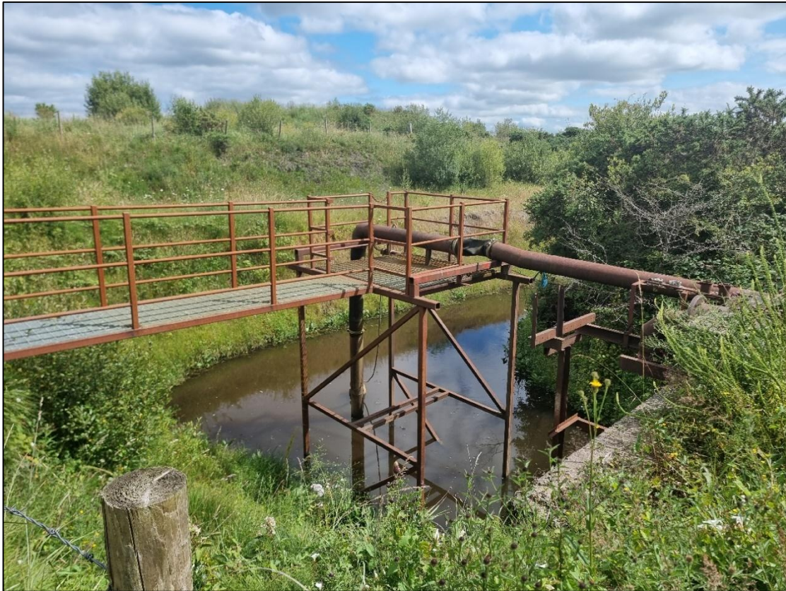
Plate 4-19 Pumping station and silt pond located in Ballydermot South Bog
